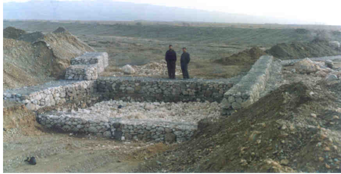
Figure 2 Gabion goal early in the intake site and Diversion Dam in aquifer Chandab
